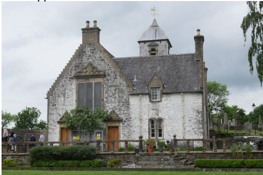
Cowane's Hospital with deteriorated limewash.
